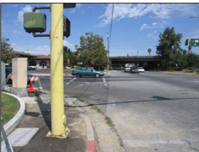
Crosswalks in poor condition and with wide turning radii at the intersection of South 7 th Street and East Virginia.
